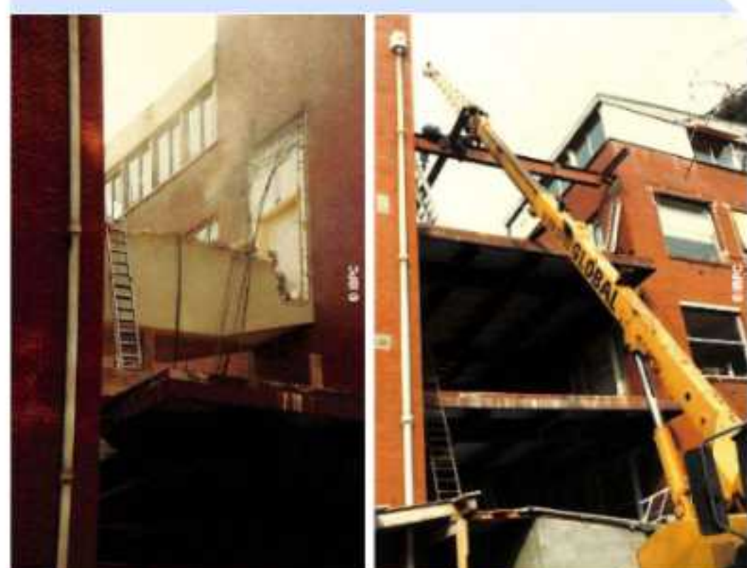
DESTRUCTION DE LA PASSERELLE DESTRUCTION OF THE AERIAL WALKWAY
